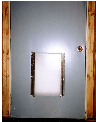
An installed closure on metal door Photo 2
