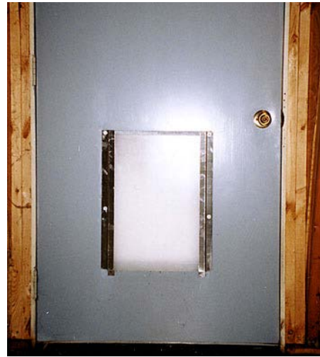
An installed closure on metal door Photo 2
